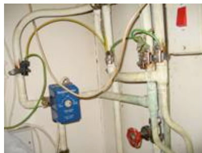
Fig. 2 Service pipes in the immersion heater cabinet where sensors were attached.
